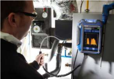
Fig. 50: Spillage test: Searching for condensate
