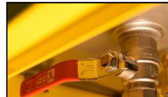
Drain Valve in Closed Position
