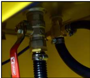
DRAIN VALVE IS OPEN (HANDLE IN VERTICAL POSITION).
