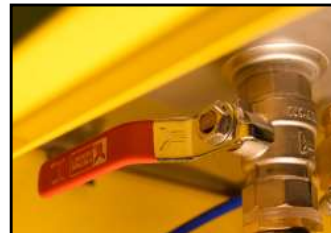
DRAIN VALVE IS CLOSED (HANDLE IN HORIZONTAL POSITION).
