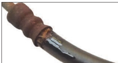
COMMON PROBLEM Leaking hose at collar
