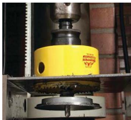
After the hole has been drilled, the core can clearly be seen at the end of the pilot drill.
