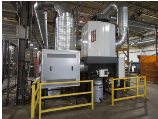
Push/Pull System installed at Elgin Sweeper Company
