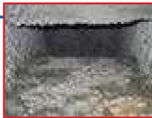
A probe's-eye view of a filthy air-conditioning duct
