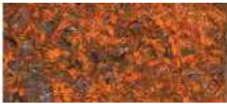
Without corrosion protection treatment
